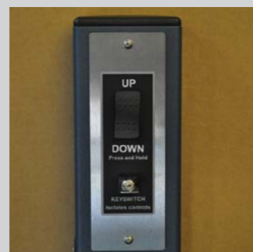
Key Switched Controls
